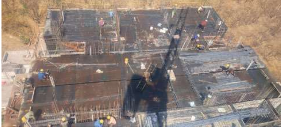
VJ INDILIFE BALANCE PORTION REINFORCEMENT BINDING IS IN PROGRESS AT 15TH FLOOR. BLOCK WORK IS IN PROGRESS AT 8TH FLOOR.
