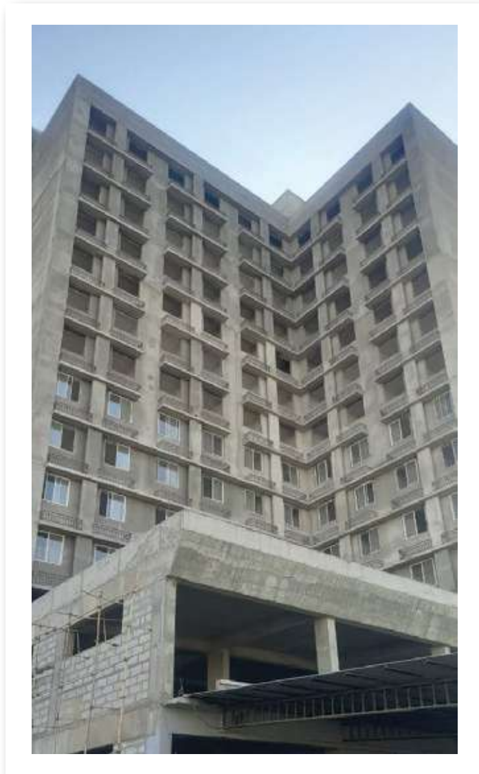
VJ TOWN CENTRE RCC WORK, BLOCK WORK & EXTERNAL PLASTER WORK IS COMPLETED.
