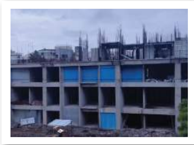
YASHWIN SUPERNOVA - 'A' 2ND-FLOOR SLAB SHUTTERING AND REINFORCEMENT BINDING WORK IS IN PROGRESS.
