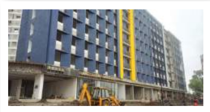
VJ HAPPINESS STREET INTERNAL PAINTING WORK IS IN PROGRESS ON 3RD, 4TH AND 5TH FLOOR.
