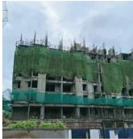
YASHWIN SUPERNOVA - 'C' 7TH FLOOR SLAB SHUTTERING AND REINFORCEMENT BINDING WORK IS IN PROGRESS.
