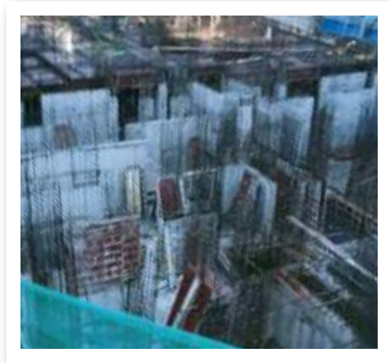
YASHWIN SUPERNOVA - 'B' GROUND FLOOR SLAB SHUTTERING AND REINFORCEMENT BINDING WORK IS IN PROGRESS.
