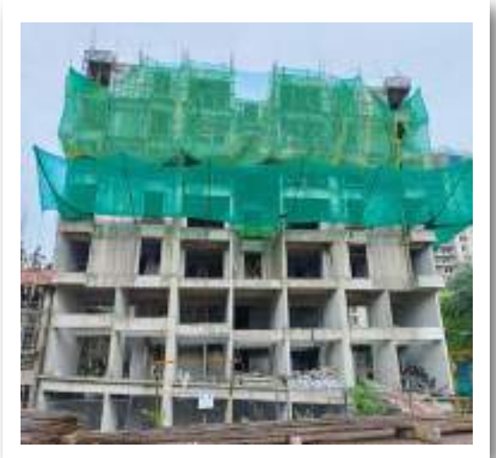
YASHONE INFINITEE - 'B1B2' 7TH FLOOR SLAB POUR - 01 READY FOR CASTING. POUR-02 SHUTTERING AND REINFORCEMENT WORK IN PROGRESS.
