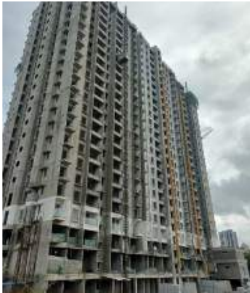
YASHWIN ORIZZONTE - 'A' OHWT- BOTTOM SLAB WORK IS IN PROGRESS. GYPSUM WORK IS IN PROGRESS AT 19TH FLOOR.
