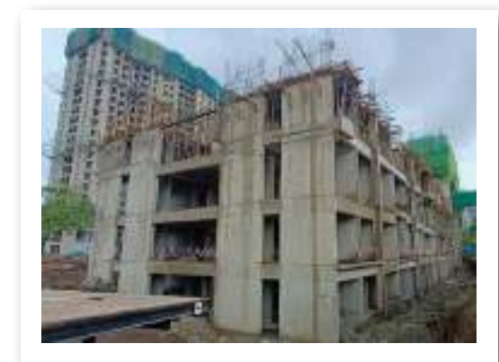
YASHONE INFINITEE - 'A1A2' 3RD FLOOR SLAB SHUTTERING AND REINFORCEMENT WORK IN PROGRESS.
