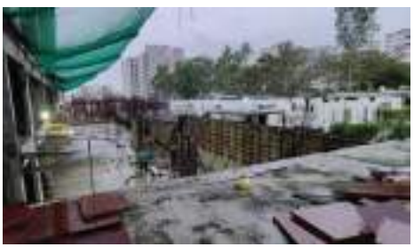
YASHWIN SUPERNOVA - 'C' PODIUM-GROUND FLOOR SLAB, RETAINING WALL AND COLUMNS CASTING IS IN PROGRESS.
