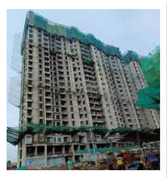
YASHONE INFINITEE - 'C1C2' PARAPET WALL, LMR AND OHWT REINFORCEMENT WORK IN PROGRESS.
