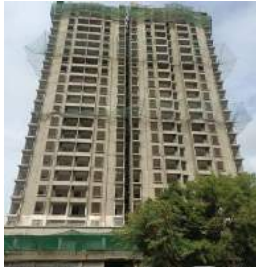
YASHWIN ORIZZONTE - 'B' OHWT- RCC WORK IS IN PROGRESS. GYPSUM WORK IS IN PROGRESS AT 18TH FLOOR.
