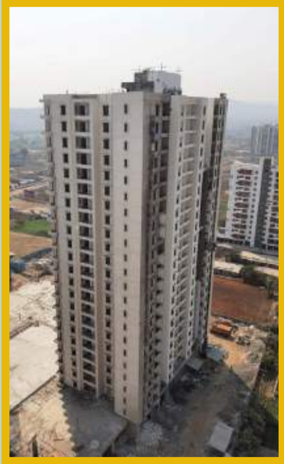
Plumbing CPVC work is in progress at 21st floor. Fire fighting work is in progress at 22nd floor.
