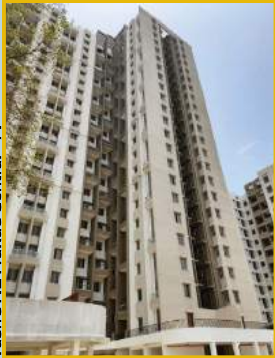
Deep cleaning 3rd to 6th Floor Completed & Lobby acid wash work 2nd to 20th Floor Completed.
