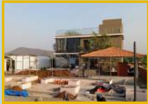
ClubHouse- Internal paint final coat work is in progress. Barbecue area flooring work is in progress.
