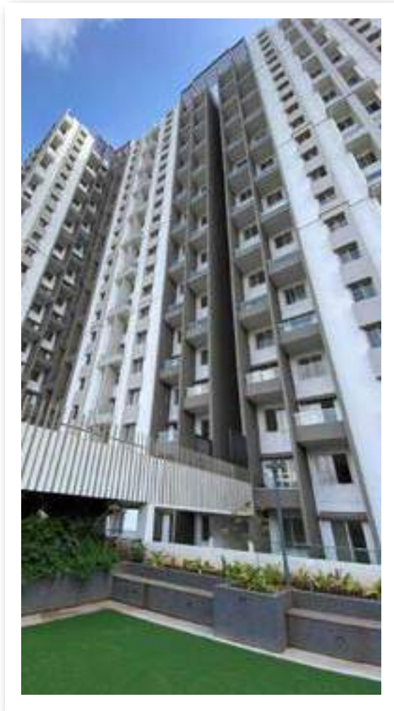
YASHONE WAKAD CENTRAL - 'D' ALUMINIUM WINDOWS FIXING WORK IS ALMOST COMPLETED. LIFT INSTALLATION WORK IS IN PROGRESS. FALSE CEILING AND GLASS DOOR FIXING WORK IS COMPLETED IN PARKING LOBBY.
