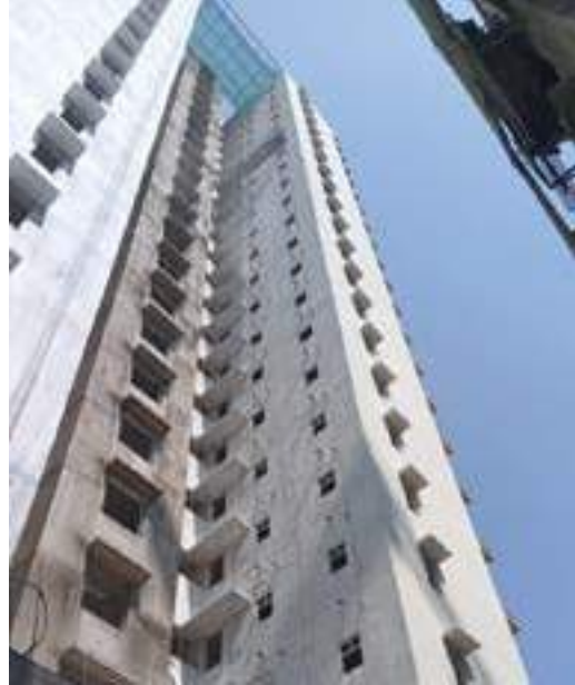
YASHWIN ORIZZONTE - 'B' ALUMINIUM WINDOWS AND DOOR FRAME FIXING WORK IS IN PROGRESS AT 12TH FLOOR. LOBBY FLOORING WORK IS IN PROGRESS AT 10TH FLOOR.
