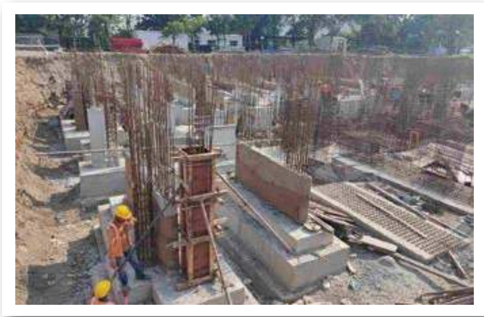
YASHONE ETERNITEE - 'C' FOOTINGS WORK AND SHEAR WALL WORK IS IN PROGRESS.
