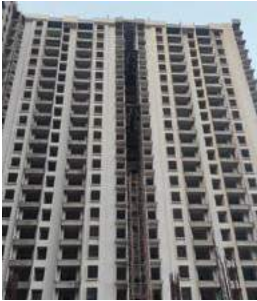
YASHWIN ORIZZONTE - 'A' FLAT FLOORING WORK IS IN PROGRESS AT 18TH FLOOR. INTERNAL WIRING WORK IS IN PROGRESS AT 12TH FLOOR. PLUMBING DUCT- EXTERNAL TEXTURE WORK IS IN PROGRESS.
