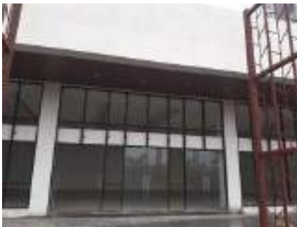
YashONE Hinjawadi - Multipurpose hall glass cladding & glass door fixing work is in progress.
