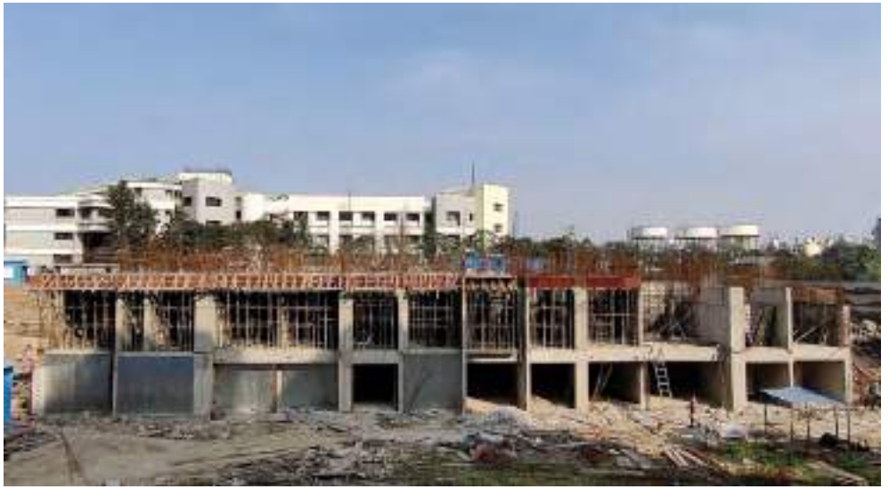
Yashwin Supernova 'A' - 2 nd slab Pour 1- slab casting work has been completed & 2 nd Pour beam shuttering work is in progress.
