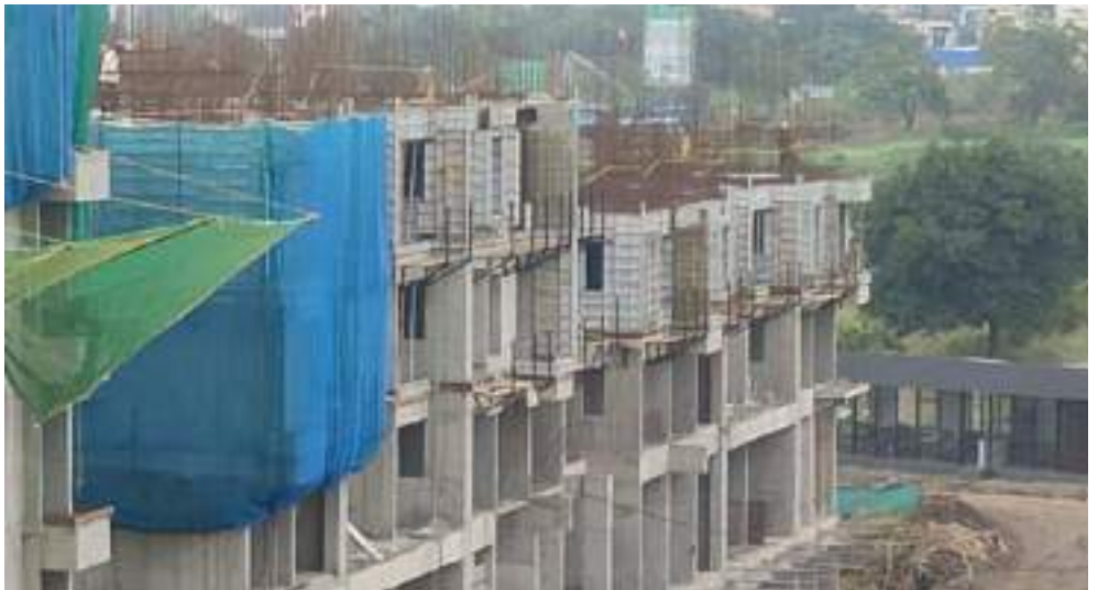
YashONE Infinitee 'C1C2' - 3 rd floor slab casting work has been completed. 4 th floor slab shuttering & reinforcement work is in progress.
