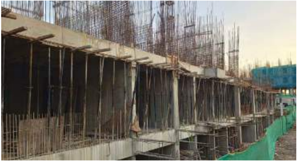
YashONE Infinitee 'B1B2' - 2 nd floor slab shearwall reinforcement and casting work is in progress.
