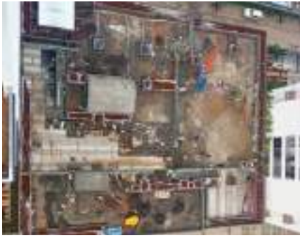
Yashwin Encore - CENTRAL PODIUM Flooring & drain channel fixing work is in progress.
