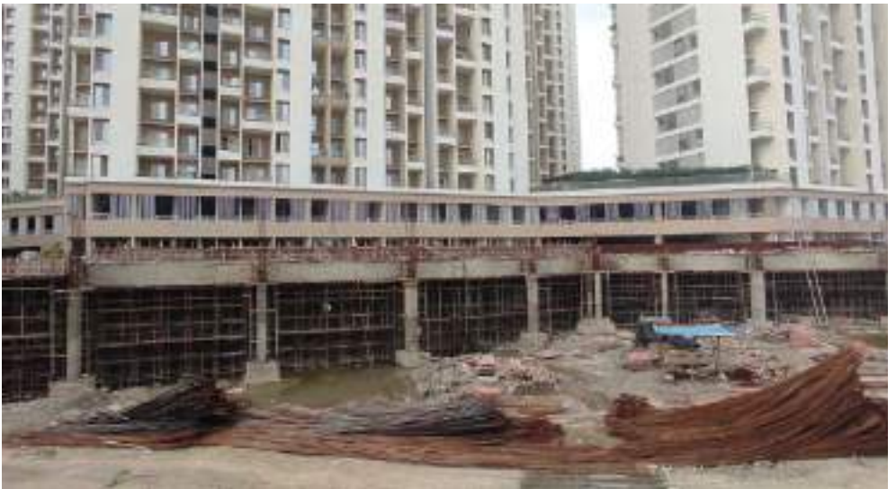
VJ HAPPINESS STREET - RHS - 1 st slab of residential parking area has been completed.
