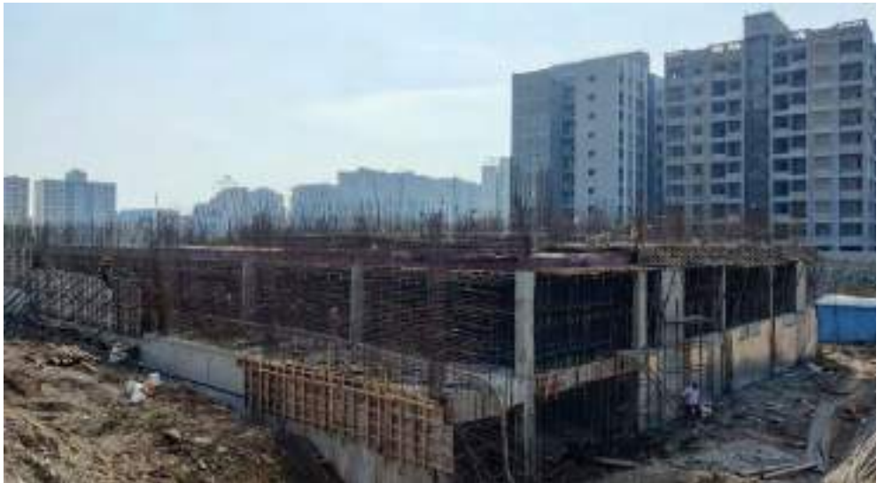
Yashwin Supernova - DEVELOPEMENT - Podium 2 nd slab retaining wall casting work & slab decking work is in progress.
