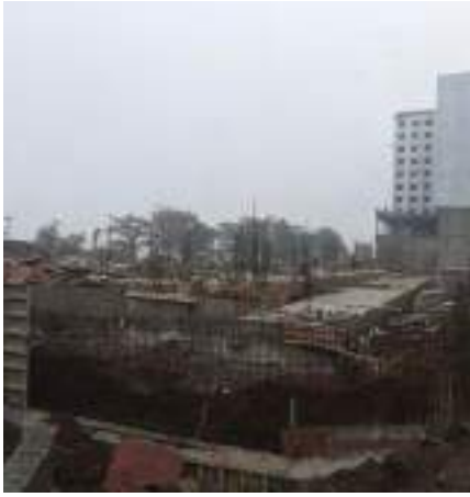
YashONE Hinjawadi - PHASE 2- Compound wall excavation work has been completed, Plumb concrete work is in progress.
