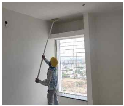
YASHWIN ENCORE - 'A2' - INTERNAL PRIMER COAT WORK IS IN PROGRESS ON 21 ST FLOOR.
