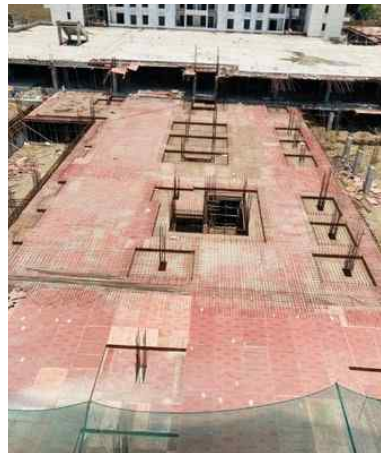
YASHONE MAAN-HINJAWADI - PODIUM PH-2 1 ST SLAB SHUTTERING & STEEL FIXING WORK HAS BEEN COMPLETED.
