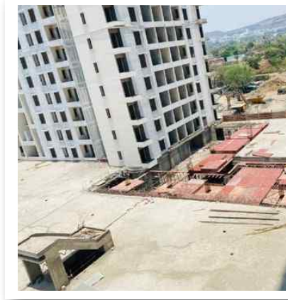
YASHONE MAAN-HINJAWADI - PODIUM PH-1 RAIN WATER SLEEVE HOLE PACKING WORK IS IN PROGRESS.
