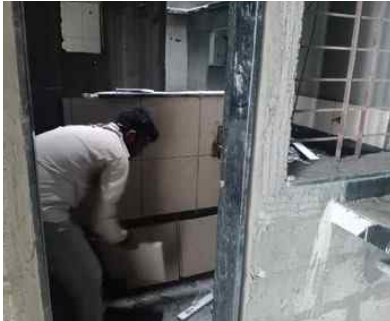
YASHWIN ENCORE - 'B1B2' DADO TILE WORK IS IN PROGRESS ON 6 TH FLOOR.
