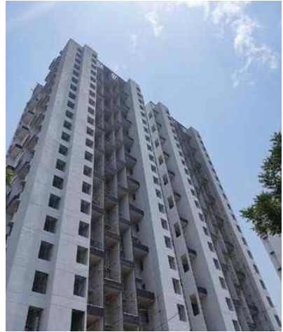
YASHWIN ENCORE - 'A2' SOUTH SIDE EXTERNAL PAINTING FINAL COAT WORK IS IN PROGRESS.
