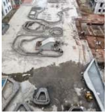
YashONE Hinjawadi 'E' - OHWT & Parapet wall work is in progress, door frame fixing work is in progress on 8 th floor.
