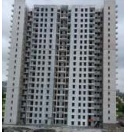
YashONE Hinjawadi 'A' - Kitchen & toilet dado tile fixing work is in progress on 16 th floor, Internal flooring work is in progress on 15 th floor.
