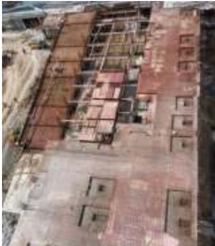
YashONE Hinjawadi - PODIUM PH-2 Ramp casting work is in progress, swimming pool slab shuttering work is in progress.
