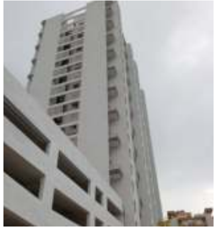
Yashwin Encore 'A2' - Internal final coat painting work is in progress, CP fittings & deep cleaning work is in progress.
