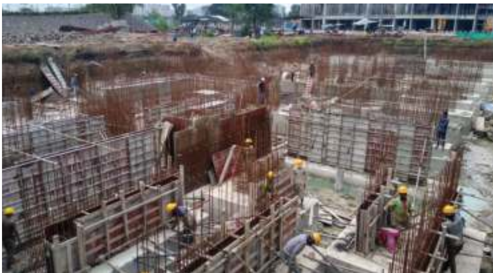
YashONE Infinitee 'B1B2' - Shearwall casting work is in progress upto plinth level.
