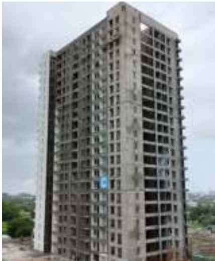
YashONE Hinjawadi 'C' - Kitchen otta fixing work is in progress on 16 th floor, wooden door frame fixing work is in progress on 16 th floor.
