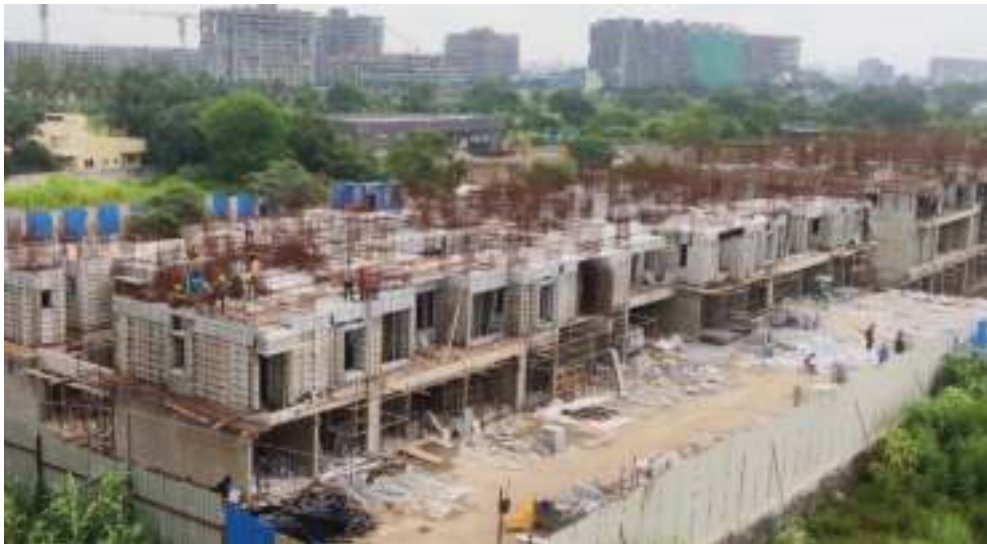
YashONE Infinitee 'D1D2' - 2 nd floor slab aluform mockup work is in progress.
