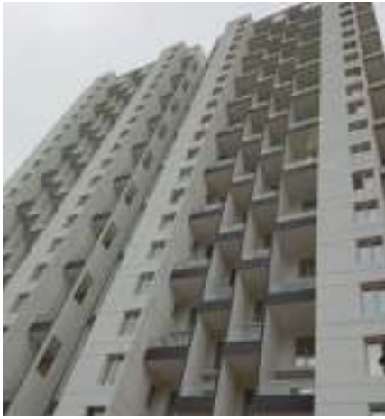
Yashwin Encore 'A1' - Internal final coat painting work is in progress, Internal CP fitting fixing work is in progress.
