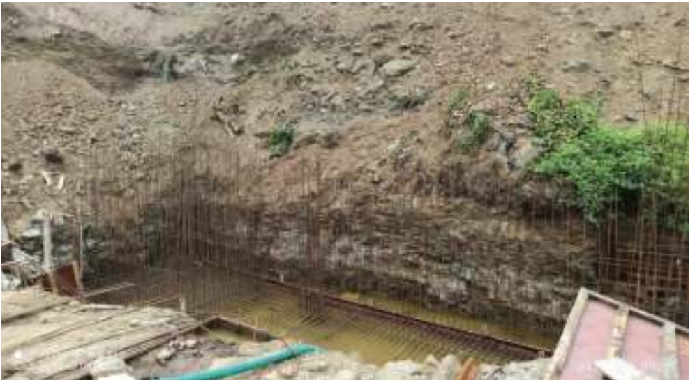
Yashwin Supernova - Subsoil drainage sump pit raft & retaining wall raft casting work is in progress.
