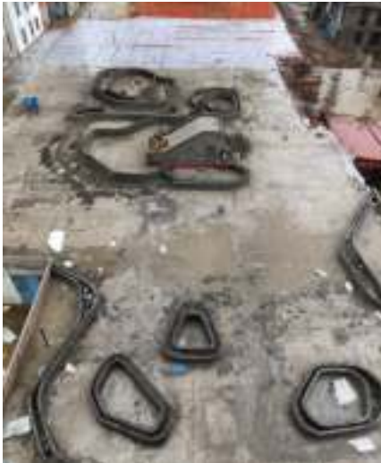
Yashone Hinjawadi - PODIUM PH -1 Planter brickwork is in progress at Pour 2, Trimix concrete work is in progress at lower parking.
