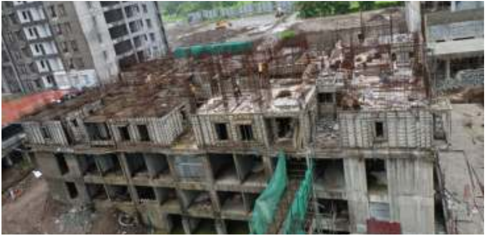
Yashone Hinjawadi 'D' - 3 rd floor slab shearwall steel fixing work is in progress.
