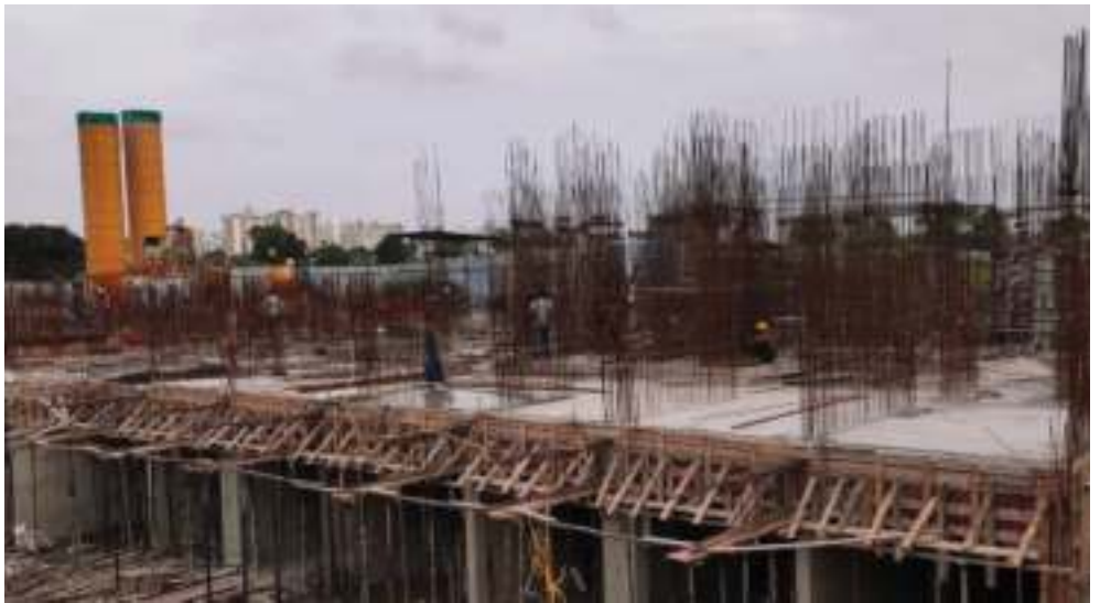
YashONE Infinitee 'D1D2' - 1 st slab shuttering & reinforcement work is in progress, 2 nd slab shearwall shuttering & reinforcement work is in progress.
