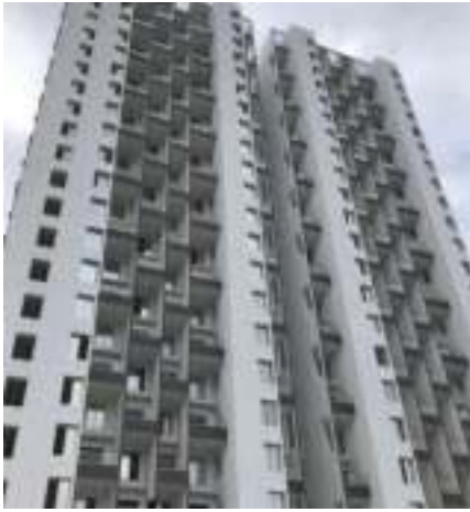
Yashwin Encore 'A1' - Glass railing fixing work is in progress, Acid wash work is in progress, External painting final coat work is in progress.
