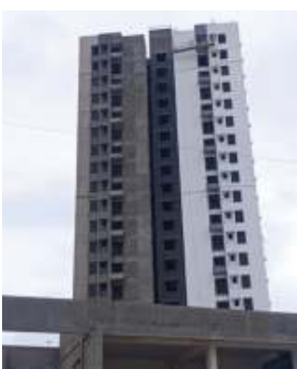
Yashwin Encore 'B1B2' - West side external painting & duct downtake work is in progress.
