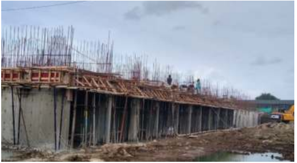
YashONE Infinitee 'C1C2' - 1 st slab casting work is in progress, Slab shuttering & reinforcement work is in progress.
