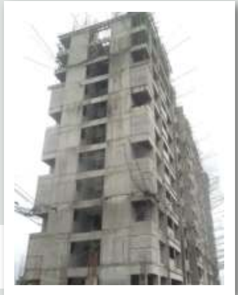
Yashwin Sukhniwas 'A' - 12 th floor slab shuttering & reinforcement work is in progress, Blockwork has been completed till 8 th floor.
