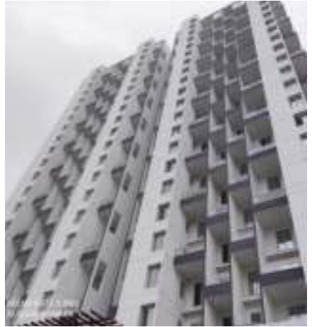
Yashwin Encore 'A2' - Glass railing fixing work is in progress, Acid wash work is in progress, Internal painting first coat work is in progress.
