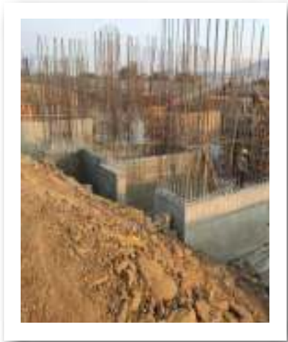
YASHWIN SUKHWIYAS - 'C' - FOOTING WORK HAS BEEN COMPLETED, SHEARWALL UPTO PLINTH HAS BEEN 70% COMPLETED, BACKFILLING WORK IS IN PROGRESS.
