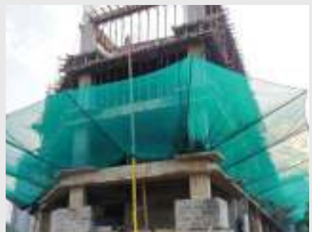
RYAN SCHOOL - A BLOCK - 5 TH SLAB COLOUMN CASTING WORK IS IN PROGRESS.
