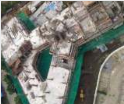
RYAN SCHOOL - A BLOCK - 5 TH SLAB COLOUMN CASTING WORK IS IN PROGRESS.
