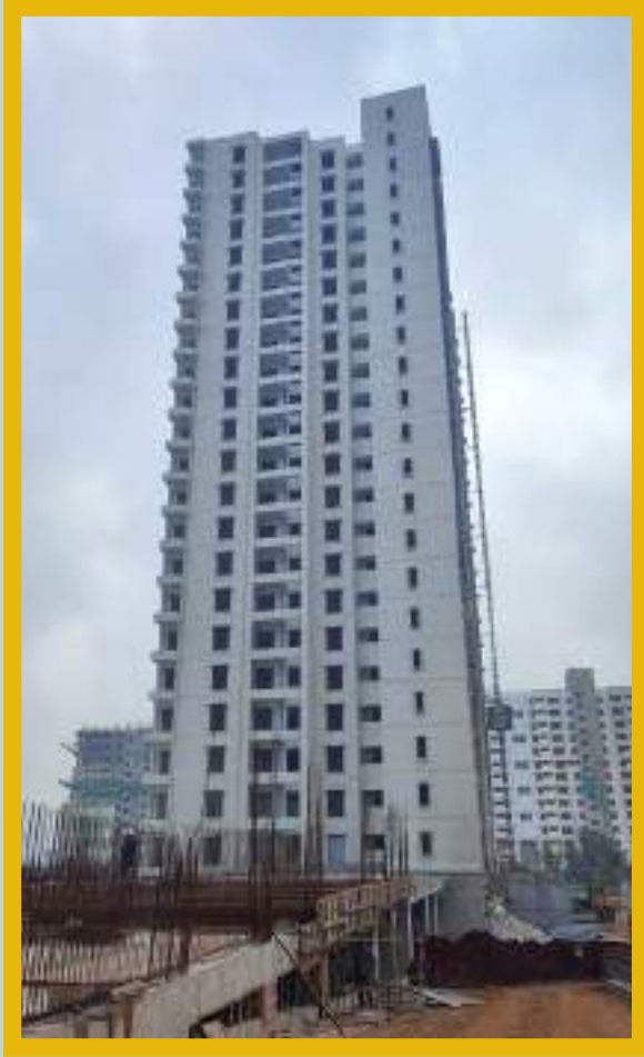
Kitchen countertop work is in progress on 22nd floor. Internal flooring work is in progress on 10th floor.
