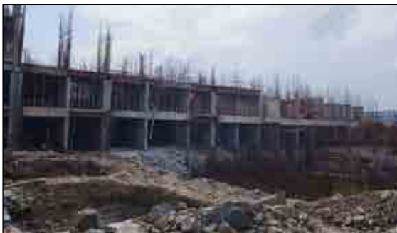
YASHWIN ENCHANTÉ - 'E1+E2' SHEAR WALL CASTING WORK IS 70% COMPLETED AT 1ST FLOOR SLAB.
