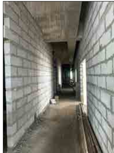
VJ HAPPINESS STREET-RHS BLOCK WORK IS IN PROGRESS OF THE 1ST FLOOR SHOPS.
