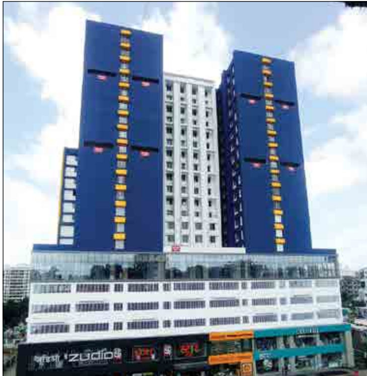
VJ GRAND CENTRAL- 2ND COAT OF EXTERNAL PAINTING WORK IS COMPLETED. FACADE WORK IS COMPLETED TILL 5TH FLOOR. FINIS FIXING WORK IS COMPLETED TILL 4TH FLOOR.
