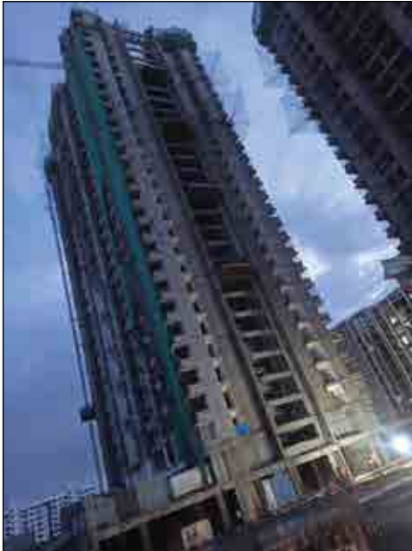
YASHWIN SUPERNOVA - 'A' GRANITE FRAME FITTING WORK IS IN PROGRESS AT 17TH FLOOR. FLOORING WORK IS IN PROGRESS AT 16TH FLOOR.
