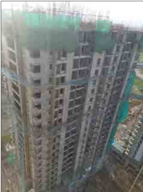
YASHWIN SUPERNOVA - 'B' FIRE FIGHTING WORK IS IN PROGRESS AT 9TH FLOOR. INTERNAL PLUMBING WORK IS IN PROGRESS AT 16TH FLOOR.
