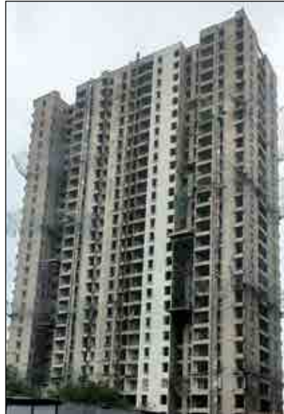
YASHONE INFINITEE - 'B1B2' WOODEN DOOR FRAME FITTING WORK IS IN PROGRESS AT 25TH FLOOR. INTERNAL PLASTER WORK IS IN PROGRESS AT 26TH FLOOR.
