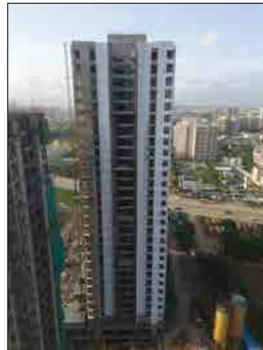
YASHWIN SUPERNOVA - 'C' KITCHEN PLATFORM WORK IS IN PROGRESS AT 27TH FLOOR. WOODEN DOOR FRAME FITTING WORK IS IN PROGRESS AT 23RD FLOOR.
