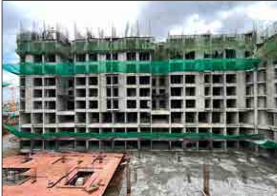
YASHWIN ENCHANTÉ - 'A1+A2' LAST POUR CASTING IS IN PROGRESS AT 8TH FLOOR SLAB.
