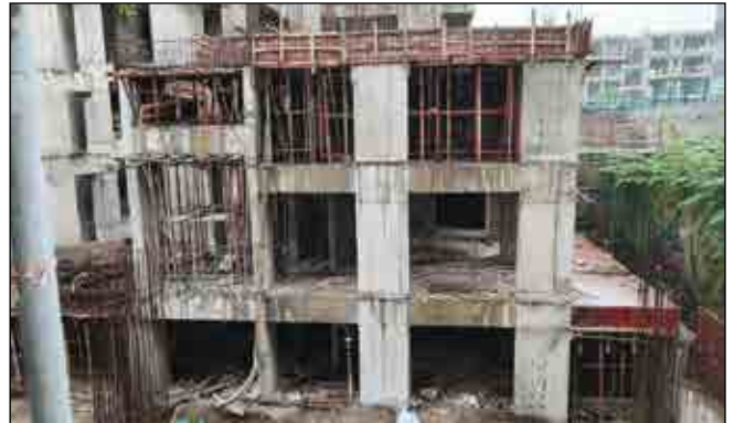
YASHWIN NUOVO CENTRO - INCLUSIVE HOUSING RCC WORK IS IN PROGRESS MEZZANINE FLOOR.
