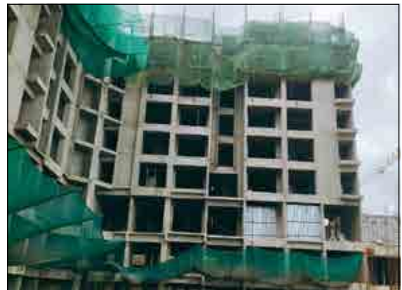
YASHWIN ENCHANTÉ - 'B1+B2' ALUFORM WORK AND REINFORCEMENT WORK IS IN PROGRESS AT 8TH FLOOR SLAB.
