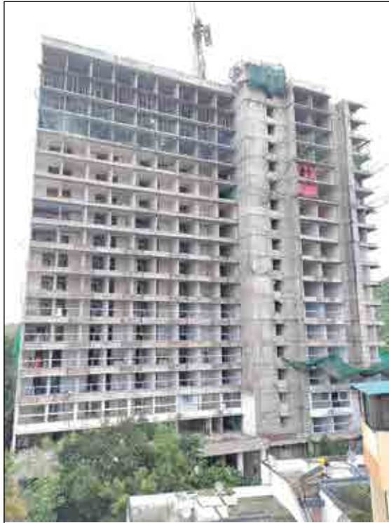
VJ INDILIFE EAST SIDE OHWT- WALL SHUTTERING WORK IS IN PROGRESS. EAST SIDE MULLION COLUMN WORK IS COMPLETED TILL 15TH FLOOR.
