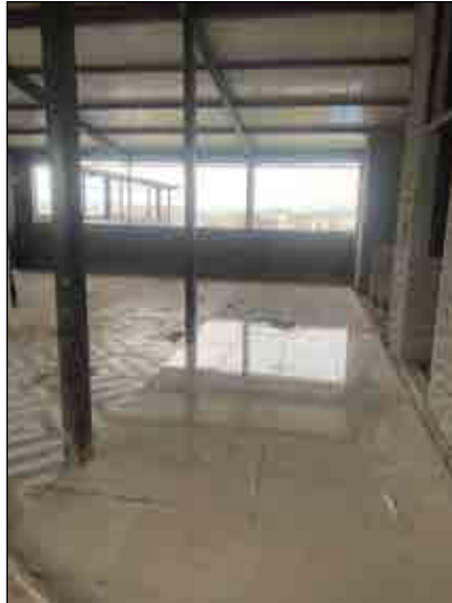
VJ TOWN CENTRE Top Terrace dining area flooring tiling work is completed.
