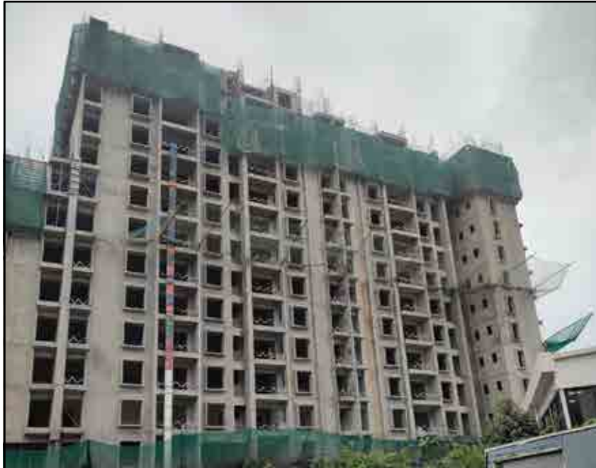
YASHONE ETERNITEE - 'D' SLAB CASTING WORK IS IN PROGRESS AT 14TH FLOOR.
