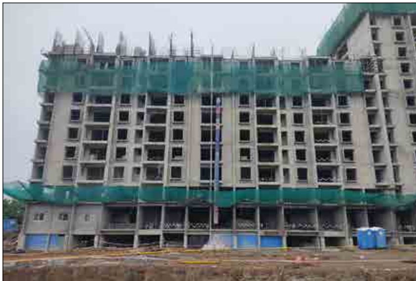
YASHONE ETERNITEE - 'C' SLAB CASTING WORK IS IN PROGRESS AT 9TH FLOOR.
