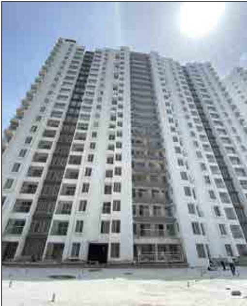
YASHONE INFINITEE - 'C1C2' TOP TERRACE WATER PROOFING WORK IS COMPLETED. GLASS RAILING FITTING WORK IS IN PROGRESS AT 21ST FLOOR.
