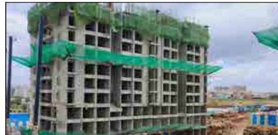
YASHWIN ENCHANTÉ - 'F1+F2' REINFORCEMENT WORK & ALUMINIUM FORM WORK IS IN PROGRESS AT 6TH FLOOR SLAB.
