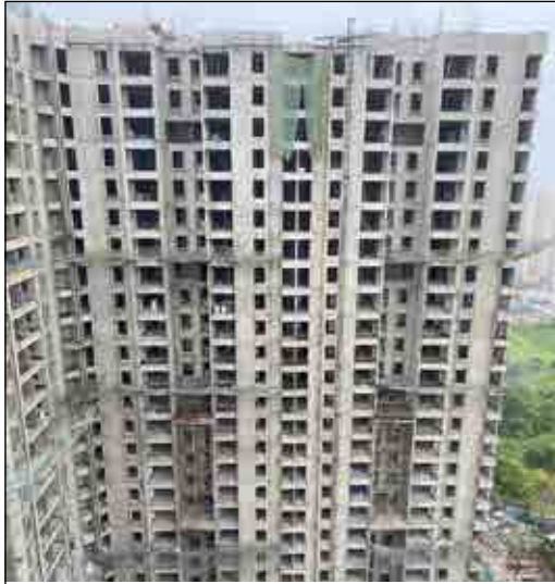
YASHONE INFINITEE - 'A1A2' BLOCKWORK IS IN PROGRESS AT 25TH FLOOR. WALL PLUMBING WORK IS IN PROGRESS AT 16TH FLOOR.
