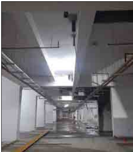
VJ HAPPINESS STREET-RHS BASEMENT- 2ND COAT PUTTY APPLICATION WORK IS IN PROGRESS.
