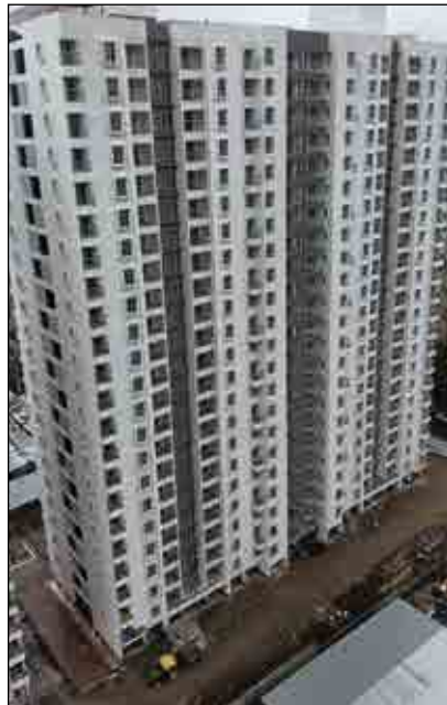
YASHONE INFINITEE - 'D1D2' INTERNAL PAINTING- 2ND COAT PAINTING WORK IS IN PROGRESS AT 22ND FLOOR. CP & SANITARY FITTING WORK IS IN PROGRESS.
