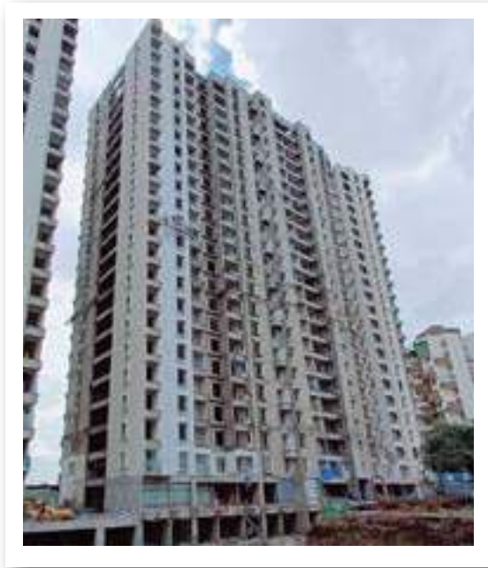
YASHONE INFINITEE - 'D1D2' INTERNAL PAINT- 2ND COAT PUTTY APPLICATION, 09TH FLOOR SLAB WORK IS IN PROGRESS.
