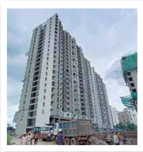
YASHONE INFINITEE - 'C1C2' INTERNAL PAINT- 2ND COAT PUTTY APPLICATION WORK IS IN PROGRESS.
