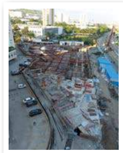
VJ HAPPINESS STREET - RHS 1ST SLAB SHUTTERING AND REINFORCEMENT WORK IS IN PROGRESS.
