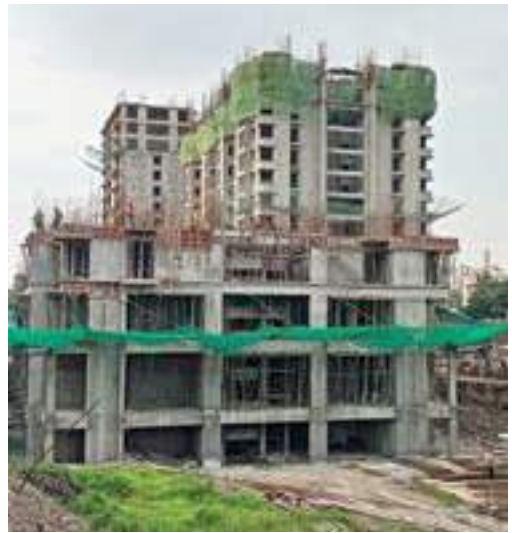
YASHWIN SUPERNOVA - 'B' 1ST FLOOR'S SLAB SHUTTERING AND REINFORCEMENT BINDING WORK IS IN PROGRESS.
