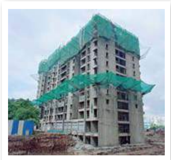
YASHONE INFINITEE - 'B1B2' 13TH FLOOR SLAB SHUTTERING AND REINFORCEMENT ALONG WITH MOCK FLOOR FINISHING WORK IS IN PROGRESS.
