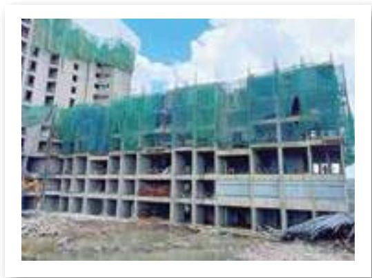
YASHONE INFINITEE - 'A1A2' 5TH FLOOR SLAB ALUFORM ERECTION WORK IS IN PROGRESS.
