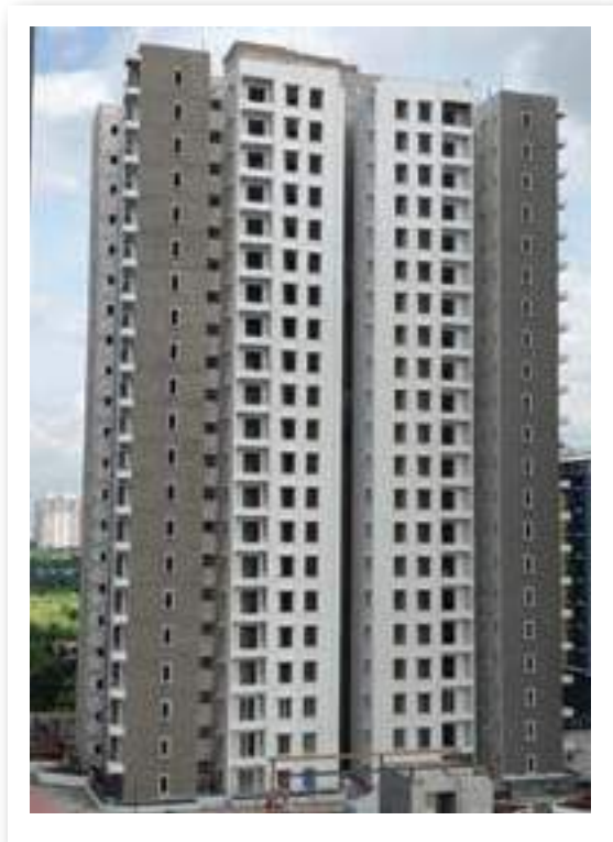
YASHONE HINJAWADI - 'D' WATERPROOFING WORK TILL 18TH FLOOR COMPLETED AND FLAT FLOORING TILL 10TH FLOOR COMPLETED. ALUMINIUM WINDOW FRAMES- 3RD FLOOR- WORK IN PROGRESS.
