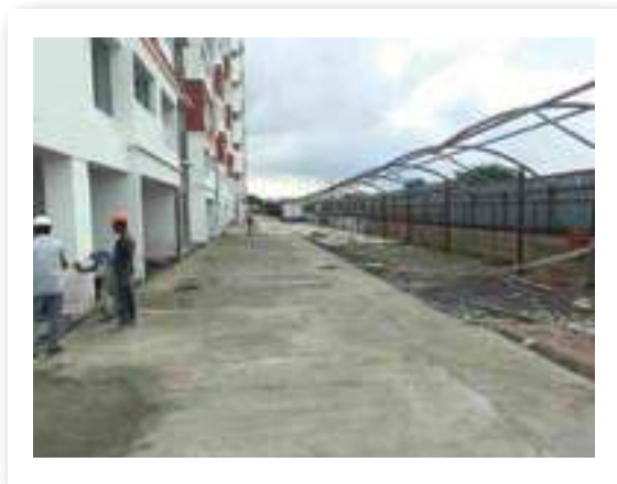
YASHWIN SUKHNIWAS PAVER BLOCK FIXING WORK IS IN PROGRESS. TRIMIX WORK IS COMPLETED.
