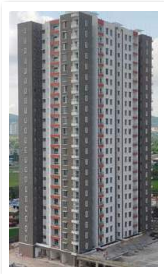
YASHONE HINJAWADI - 'E' INTERNAL PAINTING - FLATS- 2ND COAT AND CP SANITARY WORK IS IN PROGRESS.
