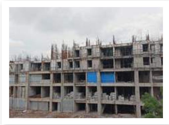
YASHWIN SUPERNOVA - 'A' 3RD FLOOR'S SLAB SHUTTERING AND REINFORCEMENT BINDING WORK IS IN PROGRESS.
