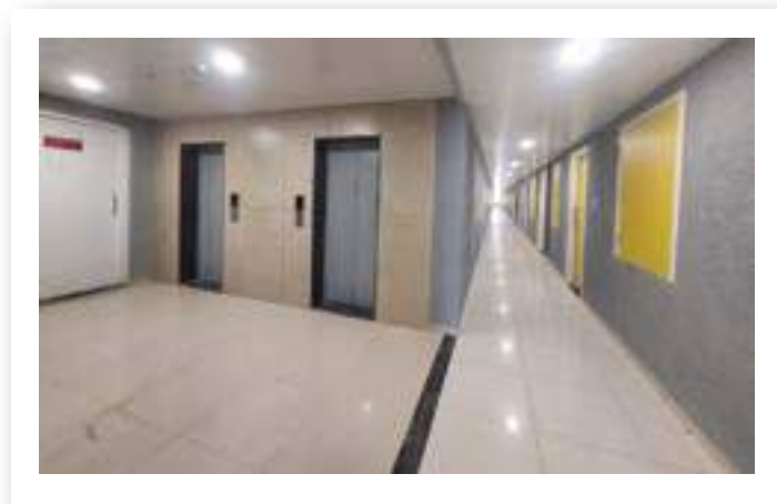
VJ HAPPINESS STREET - LHS ALL INTERNAL WORK FROM 2ND-7TH FLOOR IS COMPLETED. COMMON LOBBY WORK IS IN PROGRESS.
