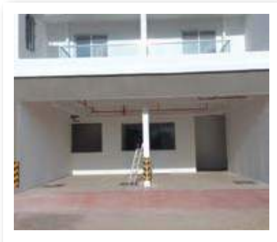
YASHONE HINJAWADI - 'E' GROUND FLOOR PARKING- 2ND COAT PAINTING WORK IS IN PROGRESS.
