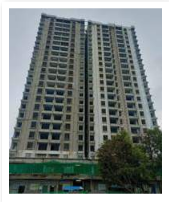
YASHWIN ORIZZONTE - 'B' FLOORING - 11TH FLOOR- WORK IS IN PROGRESS AND LOBBY FLOORING - 5TH FLOOR- WORK IS IN PROGRESS.
