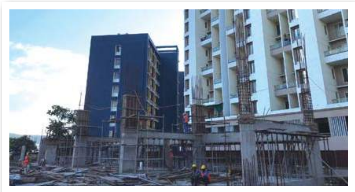
VJ HAPPINESS STREET - RHS MEZZANINE BEAM GRID CASTED COLUMN WORK IS IN PROGRESS.
