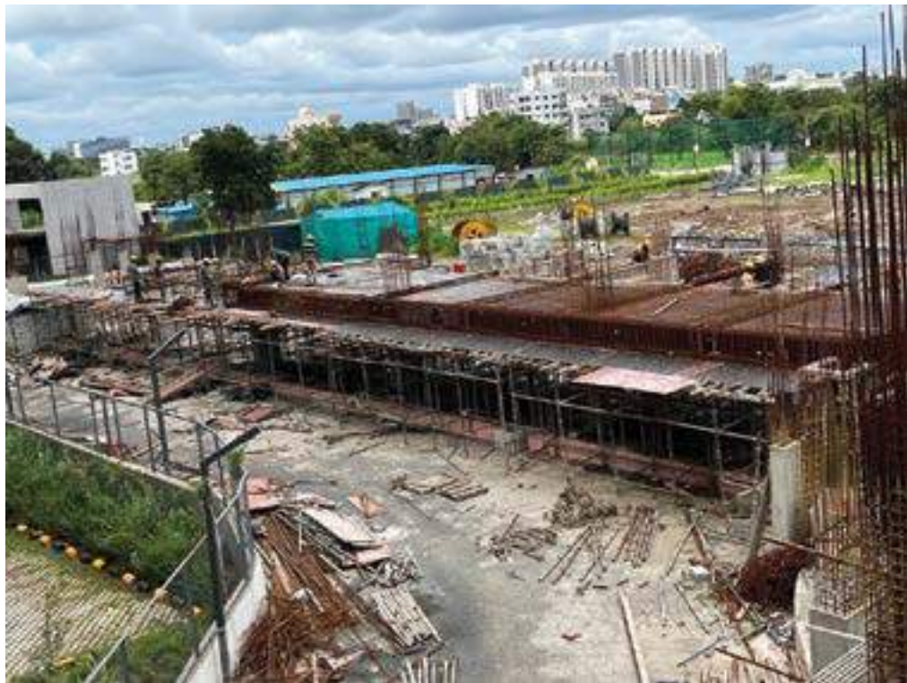
VJ ONE AVENUE Z BLOCK (SHOP AREA) MEZZANINE FLOOR SLAB SHUTTERING AND REINFORCEMENT WORK IN PROGRESS.
