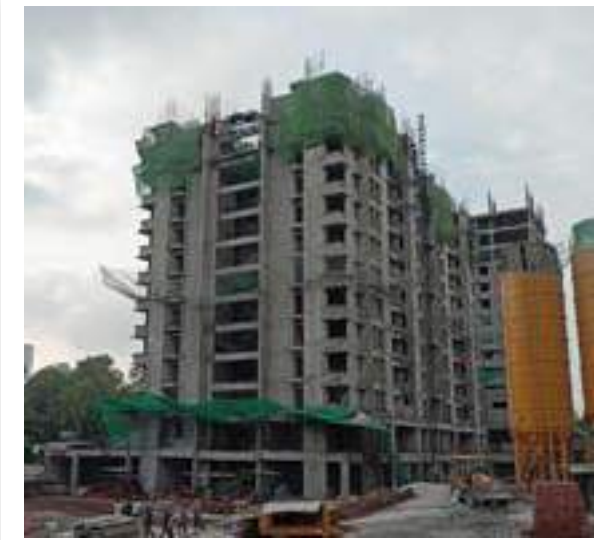
YASHWIN SUPERNOVA - 'C' 12TH FLOOR'S SLAB SHUTTERING AND REINFORCEMENT BINDING WORK IS IN PROGRESS.
