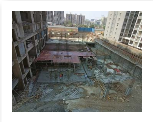
YASHWIN SUPERNOVA - EXTERNAL DEVELOPMENT A2 PODIUM - 1ST SLAB SHUTTERING AND REINFORCEMENT BINDING WORK IS IN PROGRESS.
