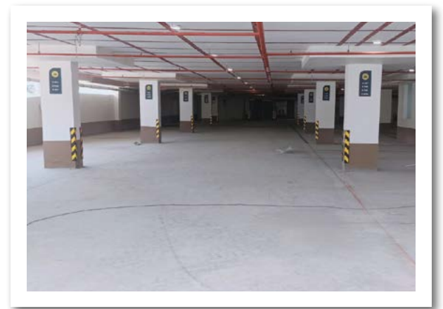
YASHONE HINJAWADI - 'D' LOWER PARKING THERMOPLASTIC PAINTING WORK IS IN PROGRESS FOR CAR PARKING.
