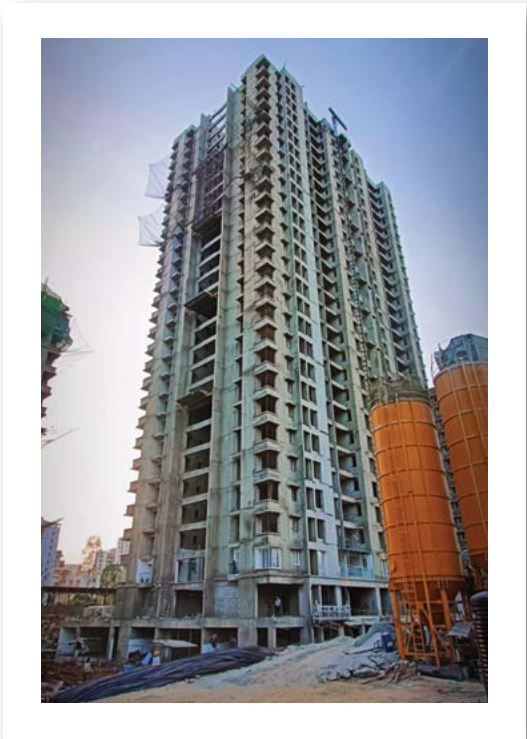
YASHWIN SUPERNOVA - 'C' OHWT & PARAPET WALL CASTING WORK IS IN PROGRESS. WOODEN DOOR FRAME FIXING WORK IS COMPLETED TILL 18TH FLOOR.
