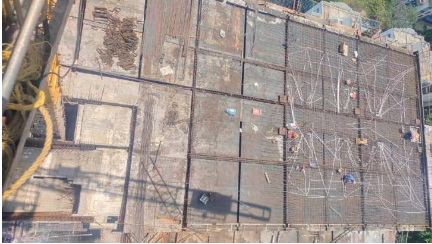
VJ INDILIFE RCC WORK - TOP TERRACE POUR 1 REINFORCEMENT BINDING WORK IS INPROGRESS.
