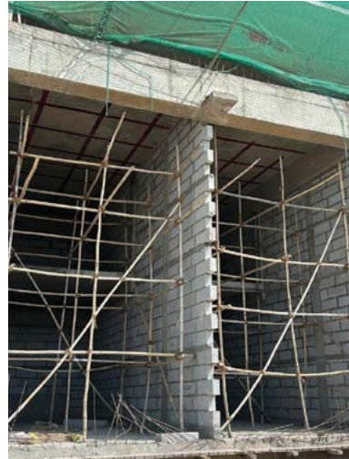
VJ HAPPINESS STREET - RHS FRONT MEGA SHOPS (GF) GYPSUM WORK IS IN PROGRESS.
