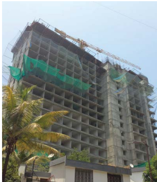
VJ INDILIFE SECONDARY CASTING - 12TH FLOOR WEST SIDE REINFORCEMENT BINDING WORK IS IN PROGRESS
