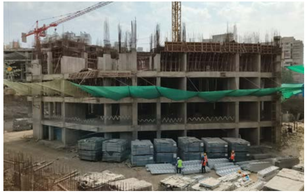
YASHWIN NUOVOCENTRO - 'A' 4TH SLAB, 1ST FLOOR RCC WORK IS IN PROGRESS.
