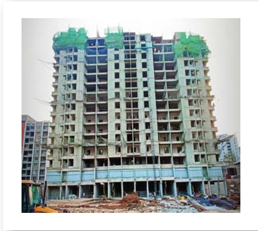
YASHWIN SUPERNOVA - 'B' 14TH FLOOR SLAB SHUTTERING AND REINFORCEMENT BINDING WORK IS IN PROGRESS. WATERPROOFING WORK IS IN PROGRESS AT 5TH FLOOR.
