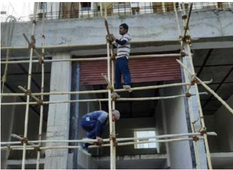
VJ HAPPINESS STREET - RHS SHOPS ROLLING SHUTTER FIXING WORK IS IN PROGRESS.
