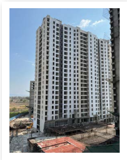
YASHONE INFINITEE - 'C1C2' INTERNAL FLAT FLOORING & LOBBY FLOORING IS COMPLETED FROM 1ST TO 22ND FLOOR.
