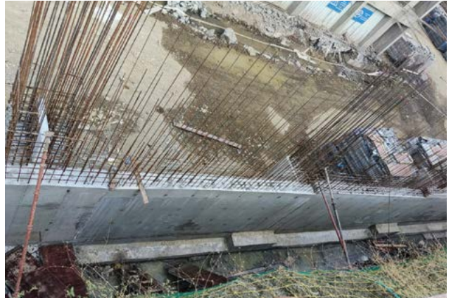
YASHWIN NUOVOCENTRO - PODIUM RETAINING WALL RCC WORK IS IN PROGRESS AT NORTH EAST CORNER.
