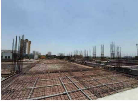
VJ HAPPINESS STREET - RHS 4TH SLAB (2ND FLOOR SLAB) SHUTTERING IS 100% COMPLETED, REINFORCEMENT WORK AND PT WORK IS IN PROGRESS.
