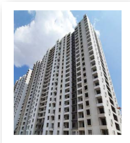
YASHONE INFINITEE - 'D1D2' DOOR SHUTTERS FIXING WORK IS COMPLETED TILL 21ST FLOOR. INTERNAL PAINTING 1ST COAT IS COMPLETED TILL 15TH FLOOR.
