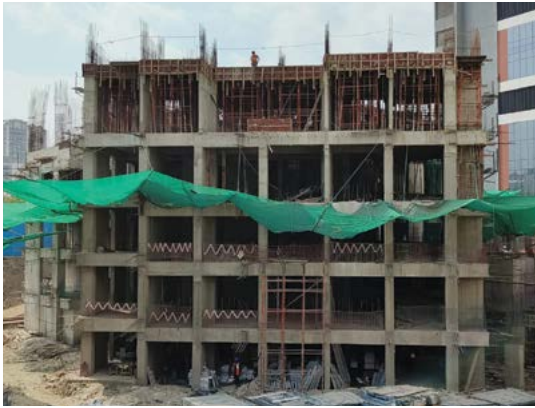
YASHWIN NUOVOCENTRO - 'B' 5TH SLAB, 2ND FLOOR RCC WORK IS IN PROGRESS.
