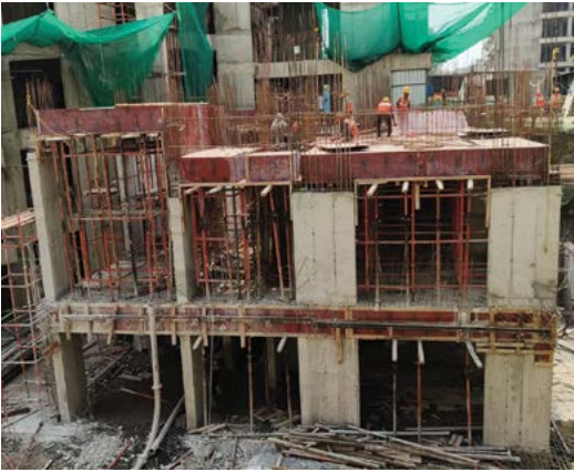
YASHWIN NUOVOCENTRO - 'IH' 2ND SLAB GROUND FLOOR RCC WORK IS IN PROGRESS.
