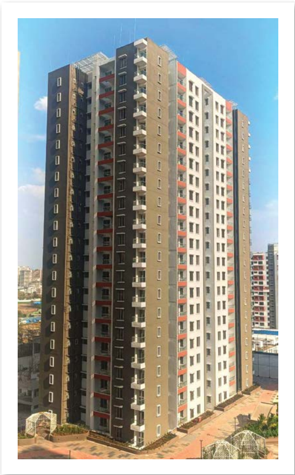
YASHONE HINJAWADI - 'D' ALUMINUM WINDOW - EXTERNAL FRAME FIXING WORK IS COMPLETED UPTO 21ST FLOOR. SANITARY FITTING WORK IS IN PROGRESS AT 21ST FLOOR.
