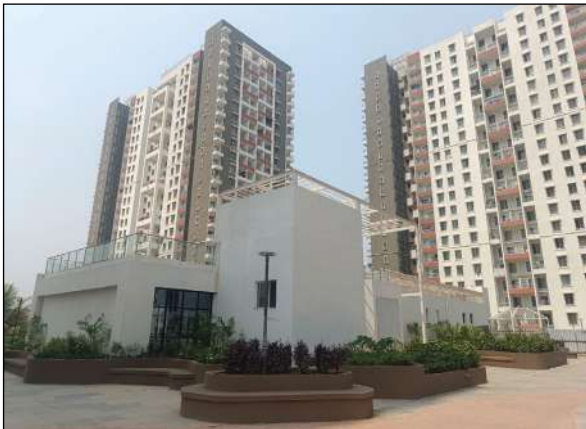
YASHONE HINJAWADI - CLUB HOUSE SECOND COAT OF EXTERNAL PAINTING IS IN PROGRESS.
