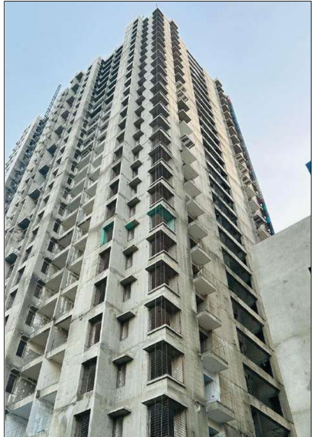
YASHWIN SUPERNOVA - 'C' GYPSUM PLASTER WORK IS IN PROGRESS AT 23RD FLOOR. WOODEN DOOR FRAME FIXING WORK IS COMPLETED TILL 19TH FLOOR.
