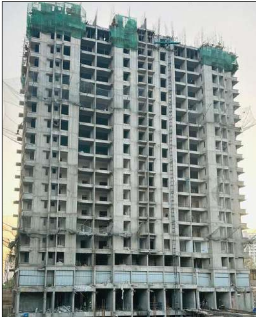
YASHWIN SUPERNOVA - 'B' KITCHEN PLATFORM FITTING WORK IS IN PROGRESS AT 10TH FLOOR. WOODEN DOOR FRAME FITTING WORK IS IN PROGRESS AT 5TH FLOOR.
