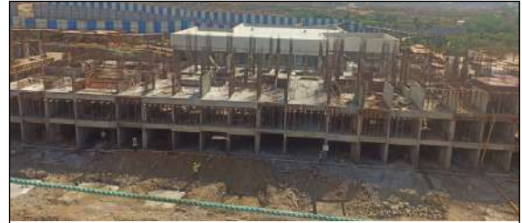
YASHWIN ENCHANTÉ - 'D1+D2' (3RD SLAB) 1ST FLOOR SLAB. 40% SHEAR WALL CASTING IS COMPLETED. SLAB SHUTTERING WORK IS IN PROGRESS.
