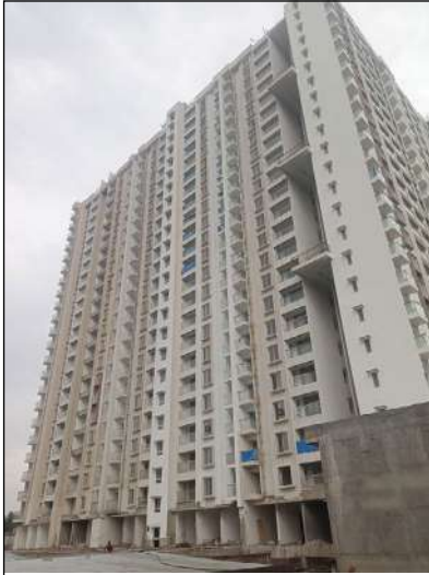
YASHWIN ORIZZONTE - 'A' ACID WASH WORK IS IN PROGRESS AT 19TH FLOOR. CP & SANITARY WARE FITTING WORK IS IN PROGRESS AT 14TH FLOOR.
