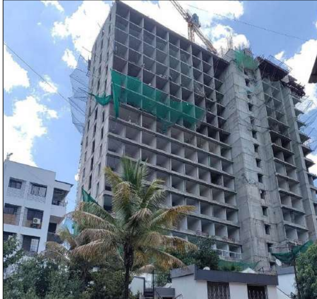
VJ INDILIFE TOP TERRACE EAST SIDE SHUTTERING IS IN PROGRESS. WATERPROOFING WORK IS IN PROGRESS AT 11TH FLOOR.
