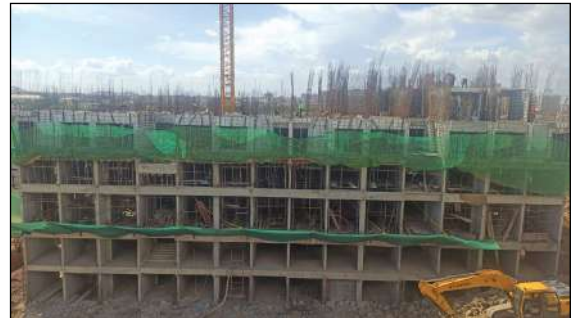
YASHWIN ENCHANTÉ - 'F1+F2' (5TH SLAB) 3RD FLOOR SLAB. 50% SLAB CASTING IS COMPLETED.
