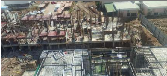
YASHWIN ENCHANTÉ - 'E1+E2' (2ND SLAB) STILT FLOOR SLAB. 60% SHEAR WALL CASTING IS COMPLETED.
