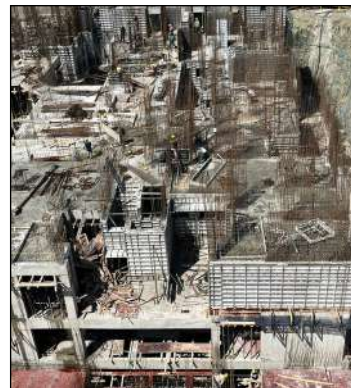
YASHWIN ENCHANTÉ - 'B1+B2' (5TH SLAB) 3RD FLOOR SLAB. ALLUMINIUM FORM WORK IS 20% COMPLETED.
