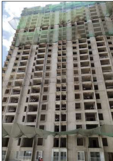
YASHWIN ORIZZONTE - 'D' GYPSUM PLASTER WORK IS IN PROGRESS AT 17TH FLOOR. FLAT FLOORING WORK IS IN PROGRESS AT 3RD FLOOR.
