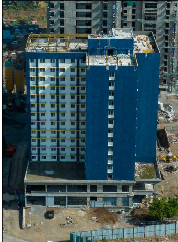
VJ TOWN CENTRE EXTERNAL PRIMER WORK IS IN PROGRESS. TOP TERRACE FABRICATION WORK IS IN PROGRESS.
