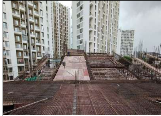
VJ HAPPINESS STREET - RHS 5TH SLAB ( SLOPING SLAB) SHUTTERING AND REINFORCEMENT WORK IS IN PROGRESS.
