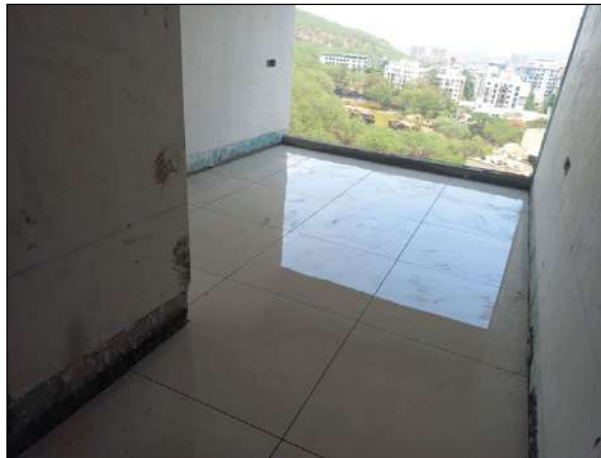
VJ INDILIFE INTERNAL UNITS FLOORING WORK IS IN PROGRESS AT 9TH FLOOR.
