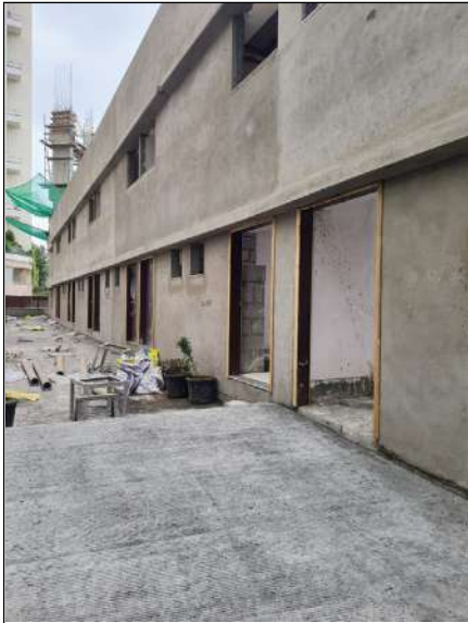
VJ HAPPINESS STREET - RHS GF BACK SIDE RETAIL SHOPS DOOR FRAME AND SHUTTER FIXING WORK IS IN PROGRESS.
