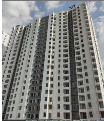
YASHONE INFINITEE - 'D1D2' KITCHEN OTA FITTING WORK IS COMPLETED FROM 1ST TO 22ND FLOOR. WATERPROOFING WORK IS COMPLETED TILL 22ND FLOOR.
