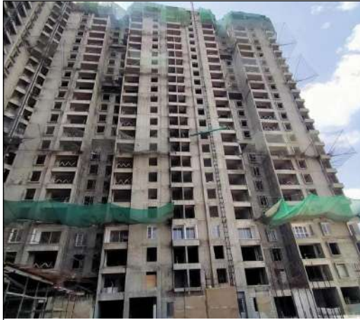
YASHONE INFINITEE - 'A1A2' GYPSUM PLASTER WORK IS COMPLETED TILL 13TH FLOOR. WATERPROOFING WITH PLUMBING WORK IS IN PROGRESS AT 11TH FLOOR.
