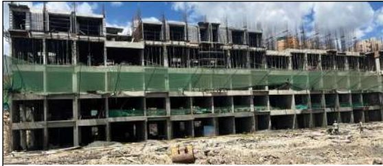
YASHWIN ENCHANTÉ - 'A1+A2' (5TH SLAB) 3RD FLOOR SLAB - 60% ALUMINIUM MOCK-UP WORK IS IN PROGRESS.
