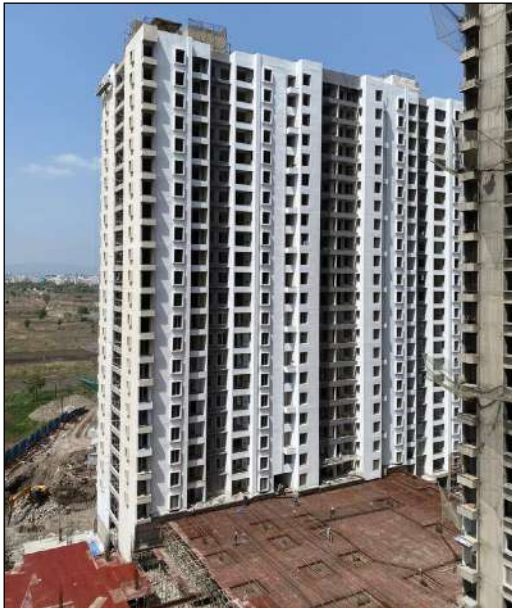
YASHONE INFINITEE - 'C1C2' DOOR SHUTTERS FIXING WORK IS COMPLETED FROM 2ND TO 22ND FLOOR. INTERNAL FLAT FLOORING IS COMPLETED FROM 1ST TO 22ND FLOOR.
