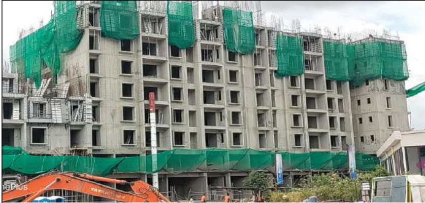
YASHONE ETERNITEE - 'D' 5TH FLOOR SLAB IS COMPLETED 6TH FLOOR SLAB SHUTTERING WORK IS IN PROGRESS.
