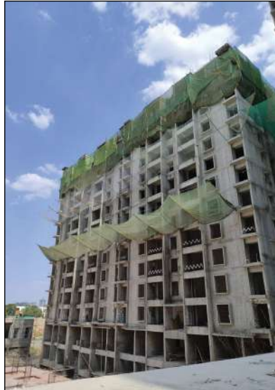
YASHWIN ORIZZONTE - 'E' AAC BLOCKWORK & PLASTER WORK IS IN PROGRESS AT 10TH FLOOR. 14TH FLOOR SLAB POUR 2 IS COMPLETED.
