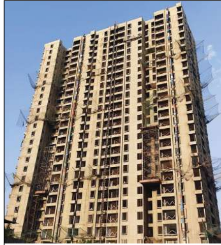
YASHONE INFINITEE - 'B1B2' BLOCK WORK IS IN PROGRESS AT 26TH FLOOR. WATERPROOFING IS COMPLETED TILL 14TH FLOOR.
