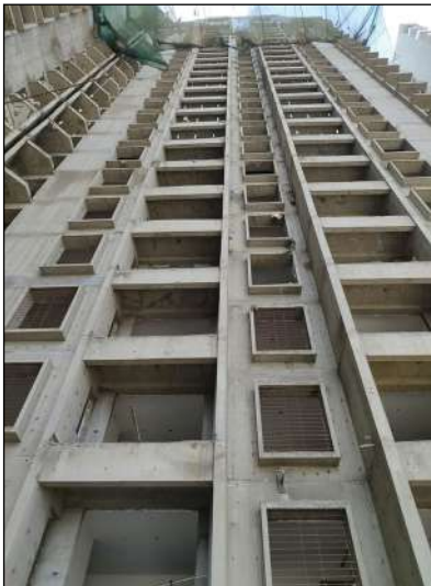
YASHWIN ORIZZONTE - 'C' AAC BLOCKWORK & PLASTER WORK IS IN PROGRESS AT 22ND FLOOR. TERRACE FLOOR SLAB WORK IS IN PROGRESS.
