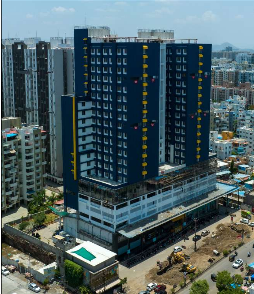
VJ GRAND CENTRAL- P1 & P2 PARKING FLOOR FINIS FIXING WORK IS IN PROGRESS. METAL FALSE CEILING IS COMPLETED UP TO 20TH FLOOR.
