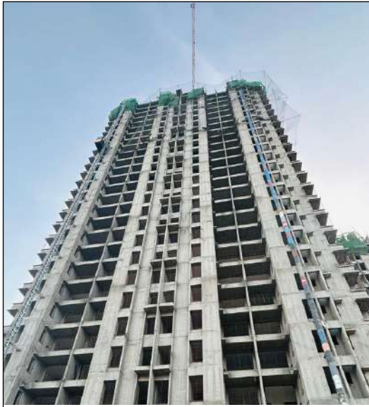
YASHWIN SUPERNOVA - 'A' GYPSUM PLASTER WORK IS IN PROGRESS AT 16TH FLOOR. FIREFIGHTING SYSTEM FITTING WORK IS IN PROGRESS AT 14TH FLOOR.
