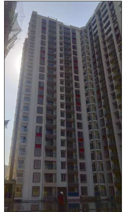
YASHWIN ORIZZONTE - 'B' CP & SANITARYWARE FIXING WORK IS IN PROGRESS AT 14TH FLOOR. EPOXY GROUTING WORK IS IN PROGRESS AT 20TH FLOOR.
